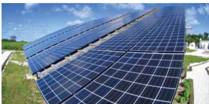
LEI Solar Power Station
